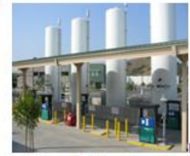
NG and LNG station, US
